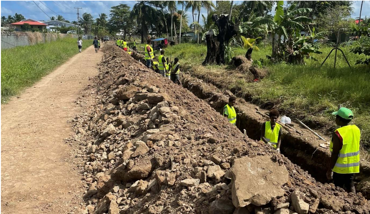
The Daru Clean Water Project mobilized the Daru community to dig the trench connecting SDP's desalination plant to Water PNG's distribution system.
